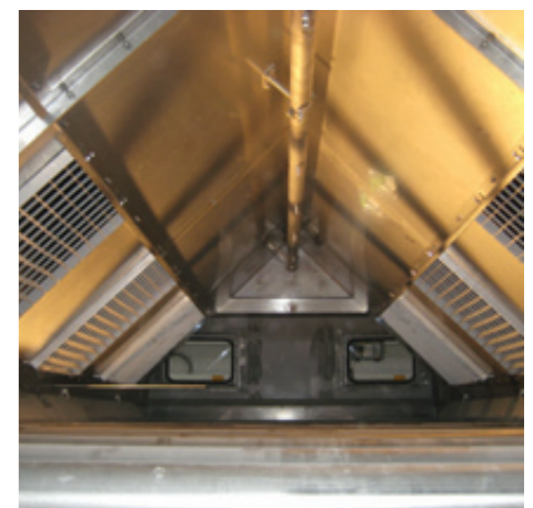
▲ Sprinkler system in a belt dryer
