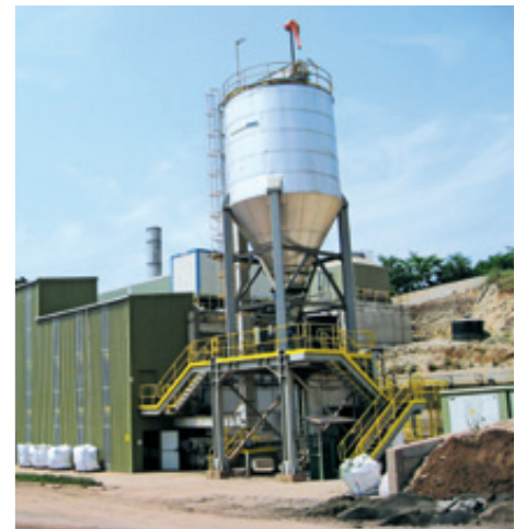
▲ Belt drying plant, Hereke, Turkey
