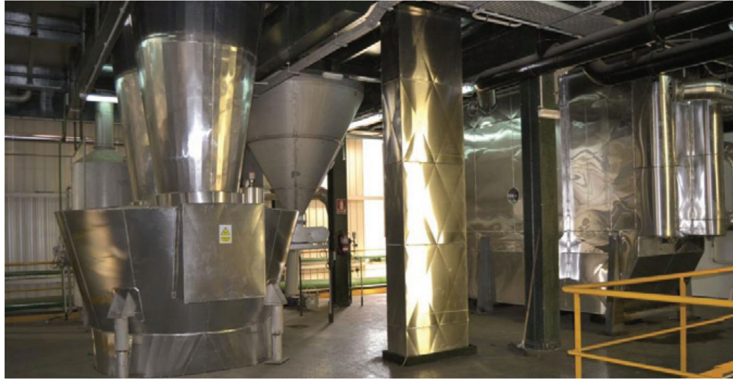
▲ Fluidized bed drying plant, Madrid, Spain
