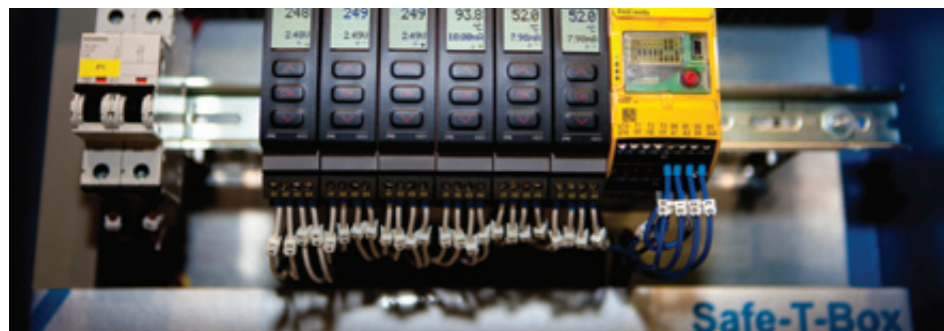
▲ Control panel of a Safe-T-Box for belt drying plants
